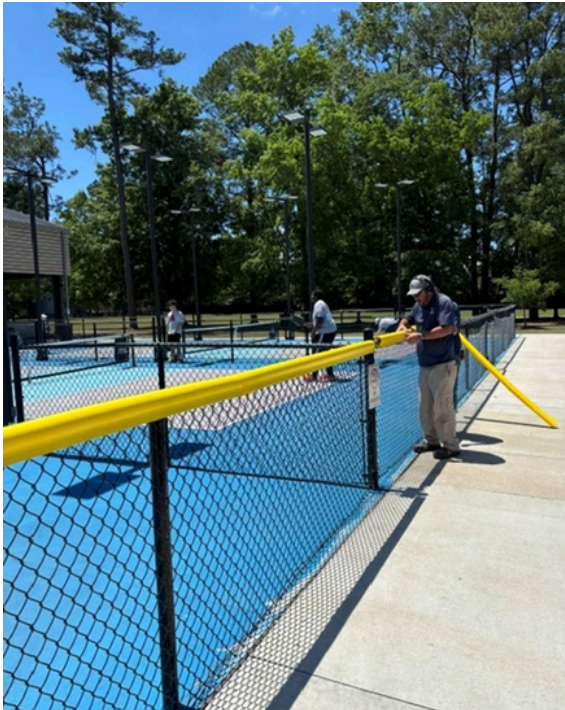
Rob La Riviere and his team installing new fence toppers at Central Creek Park Pickleball Courts
